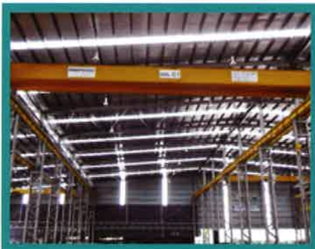
OVERHEAD CRANE (15 TONS)
