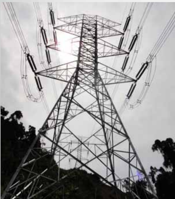
BAKUN-SIMILAJAU OVERHEAD TRANSMISSION LINE, BINTULU, SARAWAK
