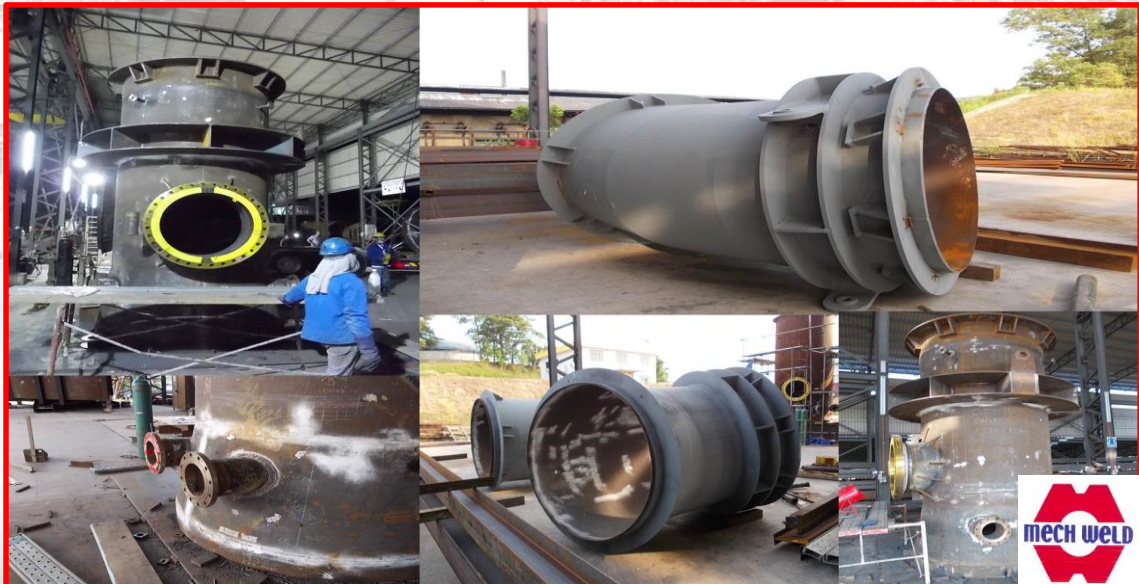
TEESSIDE EFW PROJECT OWNER : KNM PROCESS SYSTEM SDN BHD
