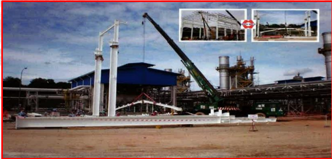
COGENERATION PROJECT, MELAKA OWNER : PETRONAS PENAPISAN (M) SDN BHD
