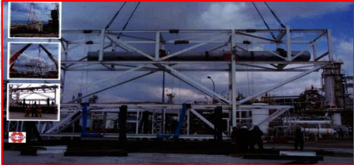
MELAKA REFINERY PSR-2 REVAMP PROJECT OWNER : MALAYSIA REFINING COMPANY SDN BHD PROJECT MANAGEMENT CONSULTANT: FOSTER WHEELER MALAYSIA
